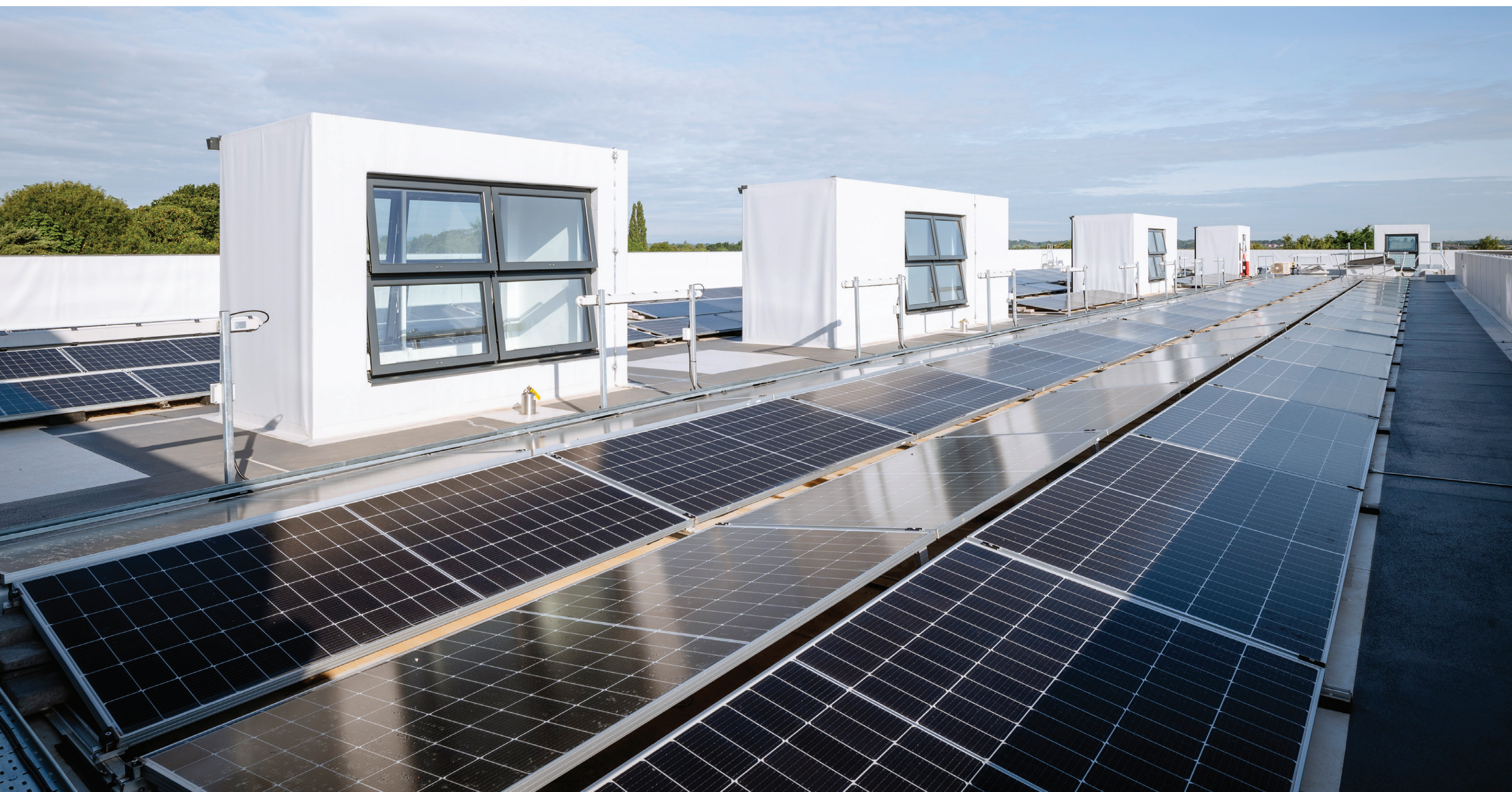
Photo showing PV panels installed by Bowmer + Kirkland at Belvidere School, Shrewsbury
